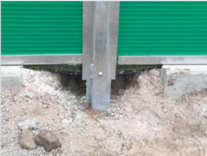
Not like this. foundations / conduits placed incorrectly.
