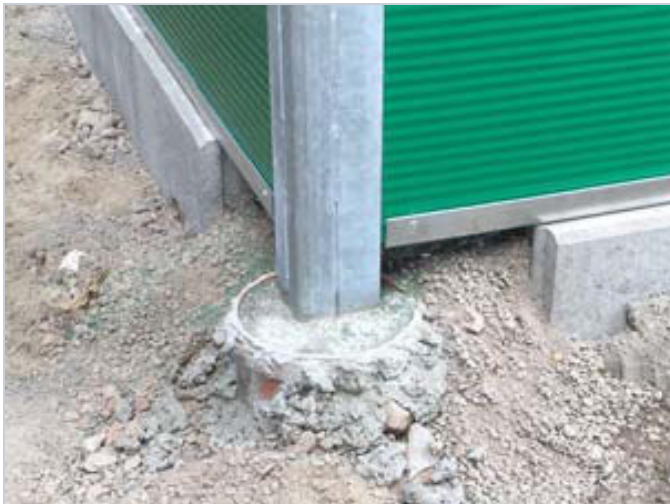
Not like this. curb not built right up to the conduit.
