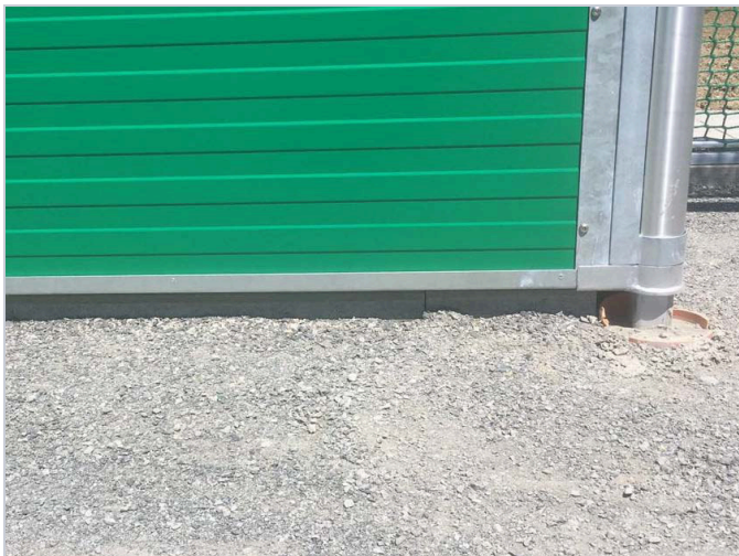
Not like this. curb not placed correctly (here too far out).
