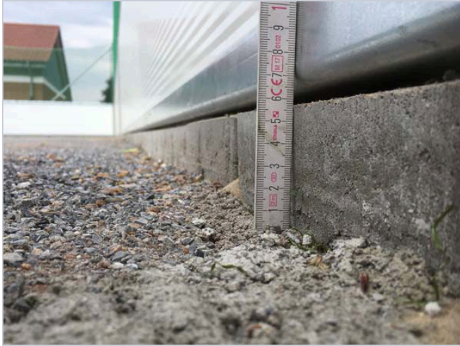
Not like this. installation height too high / low.
