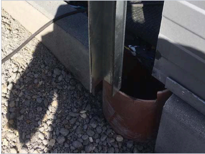
Not like this. foundation conduits too small or covered.
