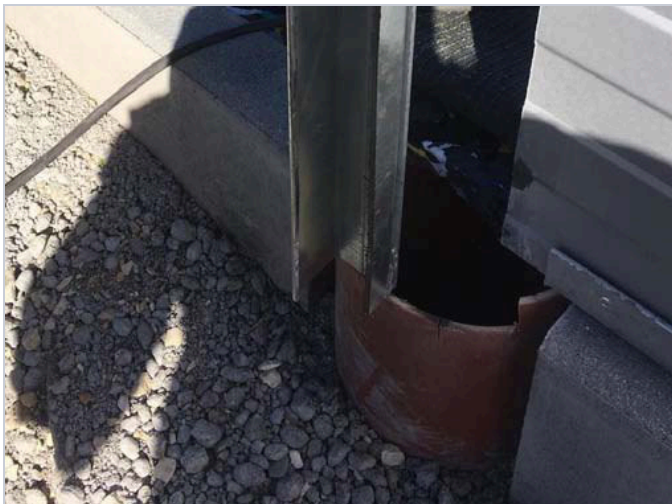
Not like this. foundations placed incorrectly.
