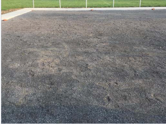
Not like this. gravel uneven / not sufficiently compacted.
