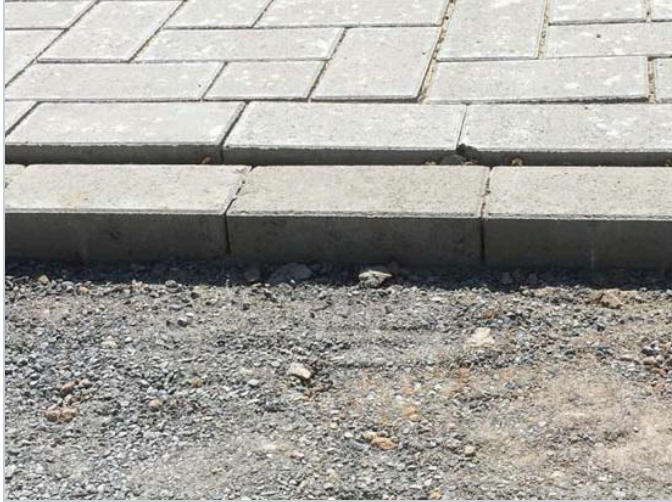
Not like this. paving stones not level with the curb.
