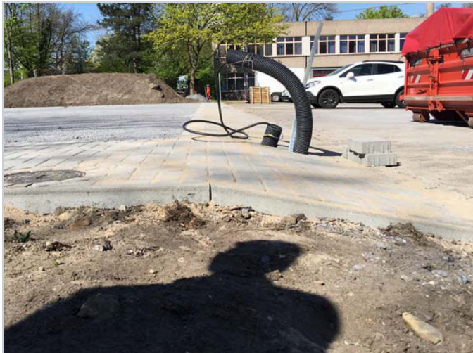
Not like this. surrounding paving sloping.
