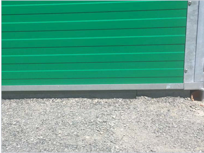
Not like this. curb not placed correctly.
